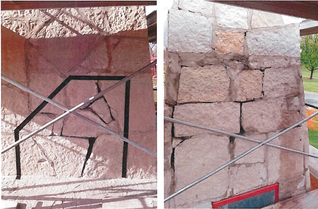
FIGURE B: During the mortar removal process we found additional stones units not attached to the backup.
