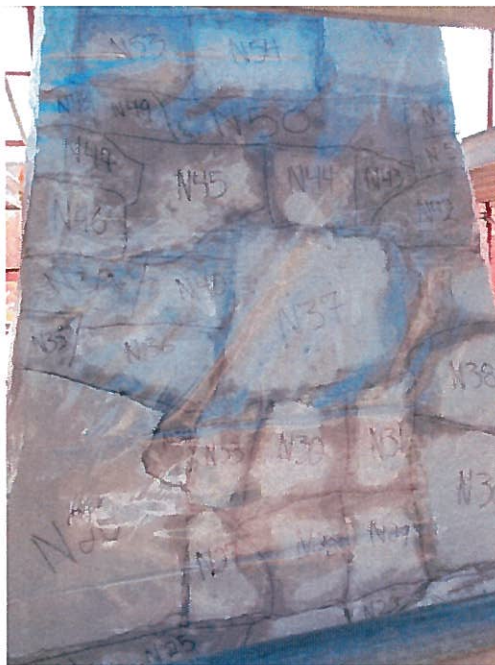
FIGURE C: Each external masonry units within the body of the obelisk was documented. This documentation will be use in the event of removal and reinstallation of individual units.
