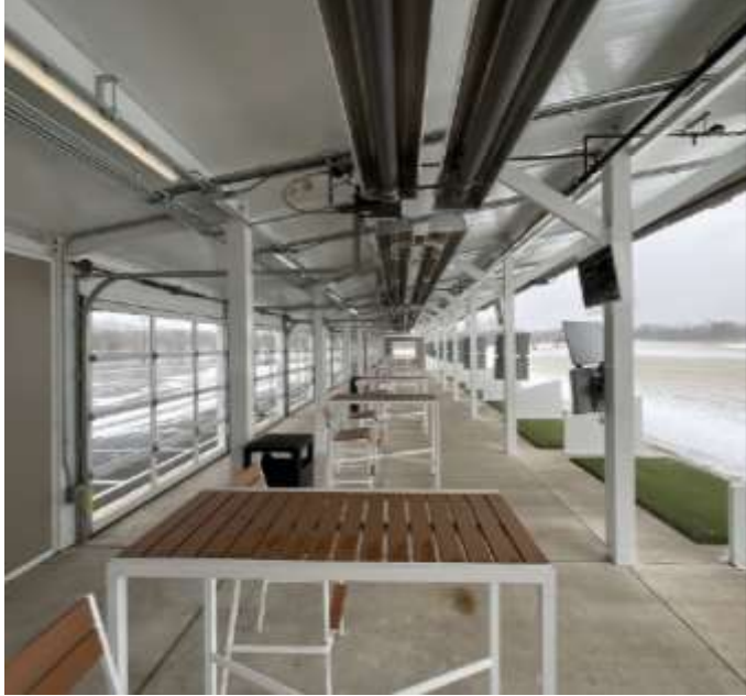
Base Bid Radiant Tube Heaters
