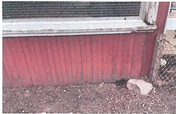
Figure 13. Deterioration of clapboards at the base of the structure
