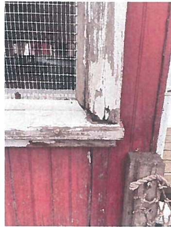
Figure 17. Deterioration at corner of opening on the south elevation
