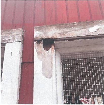
Figure 18. Damage at the frame of the opening
