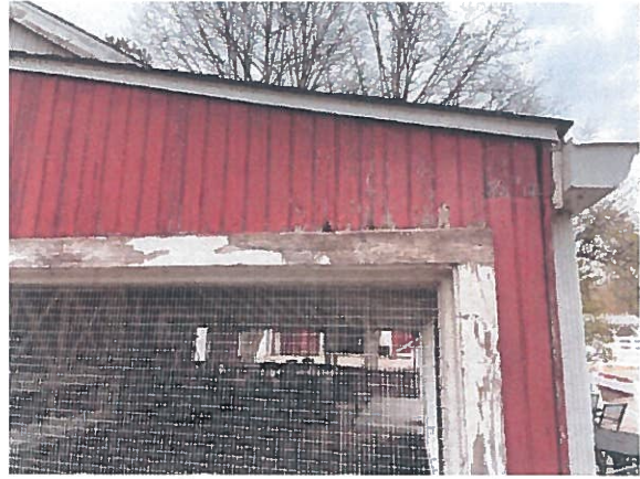
Figure 12. Deterioration at the wood clapboards and frame of the opening at south elevation
