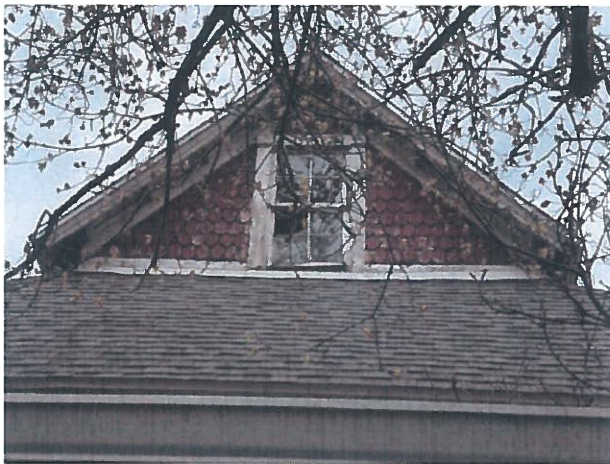
Figure 15. Upper portion view of the west elevation. Note broken windowpane.
