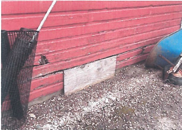
Figure 11. Deteriorated and missing clapboard on the original portion of the barn.
