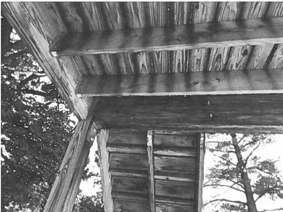
Photo 2 Rotting PSL edge beam at deck
