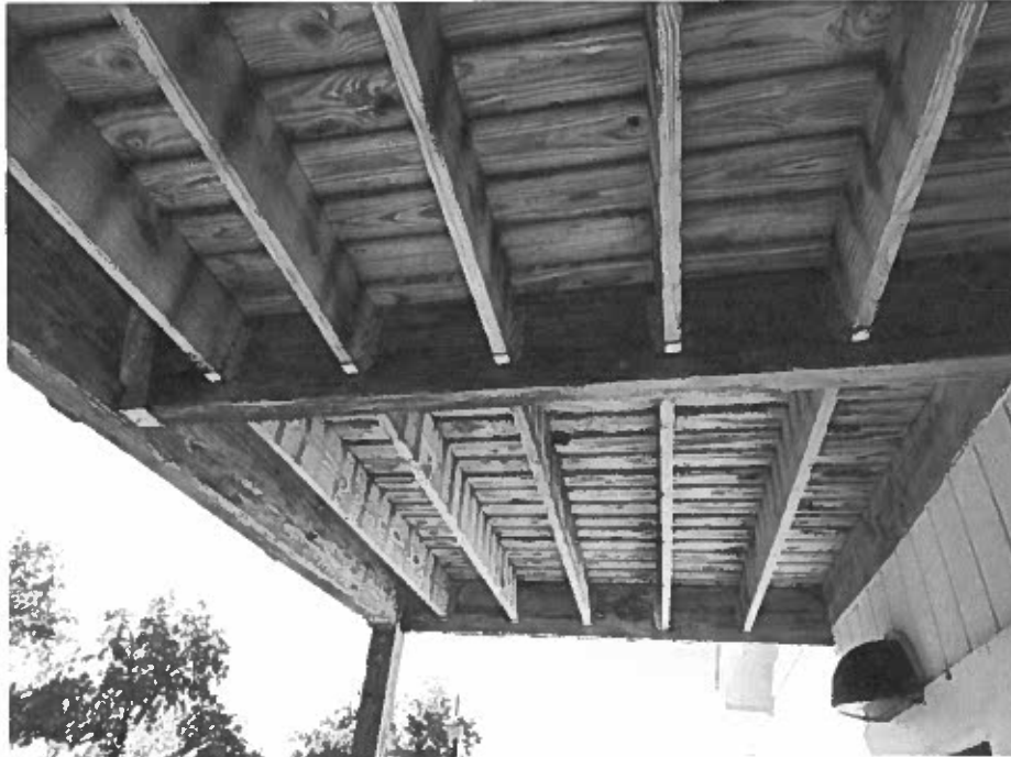
Photo 3 Rotting PSL support beam at deck
