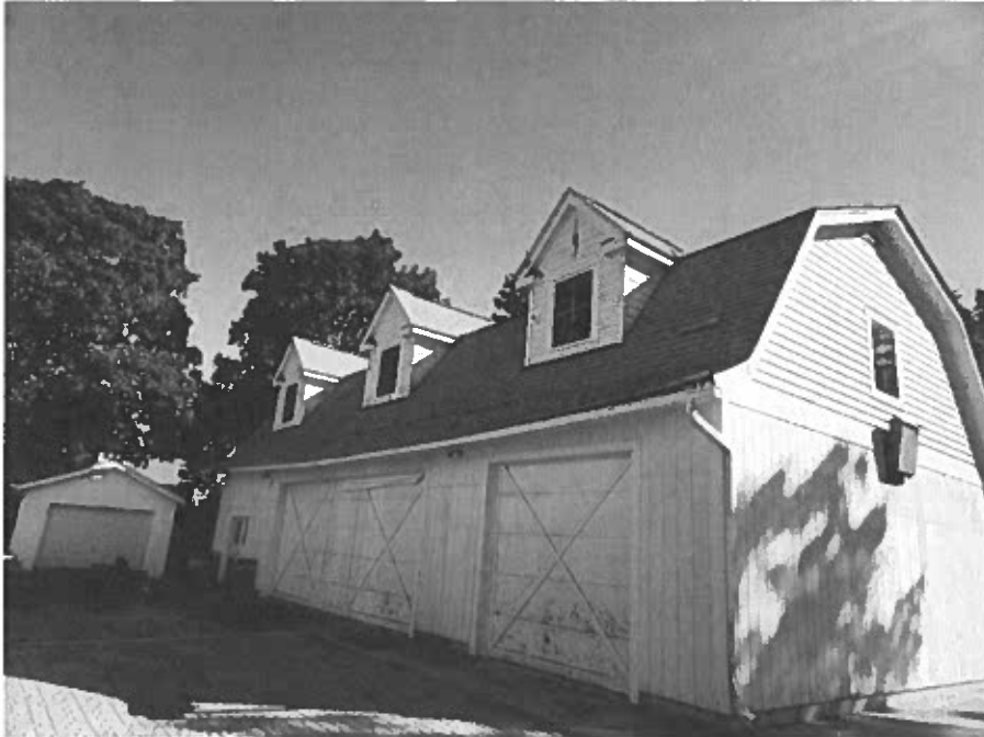
Photo 1 Sagging eave on west side of Storage Barn
